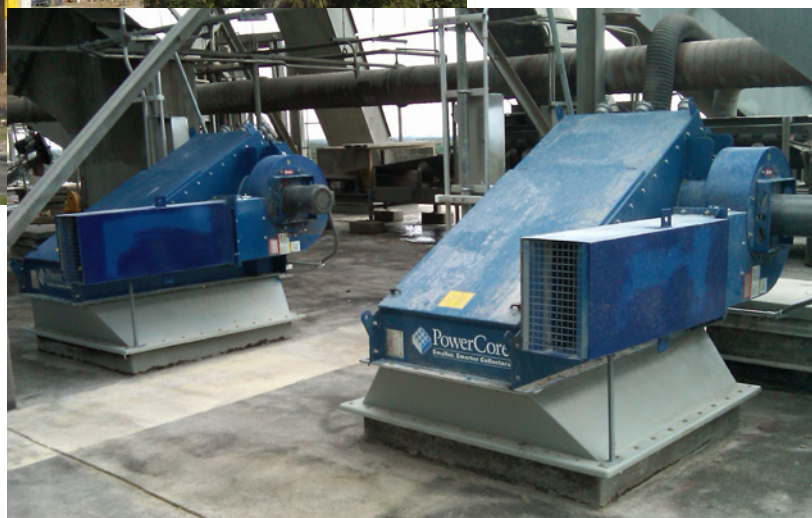
Figure 5. Point-of-Use Dust Control on Silo
