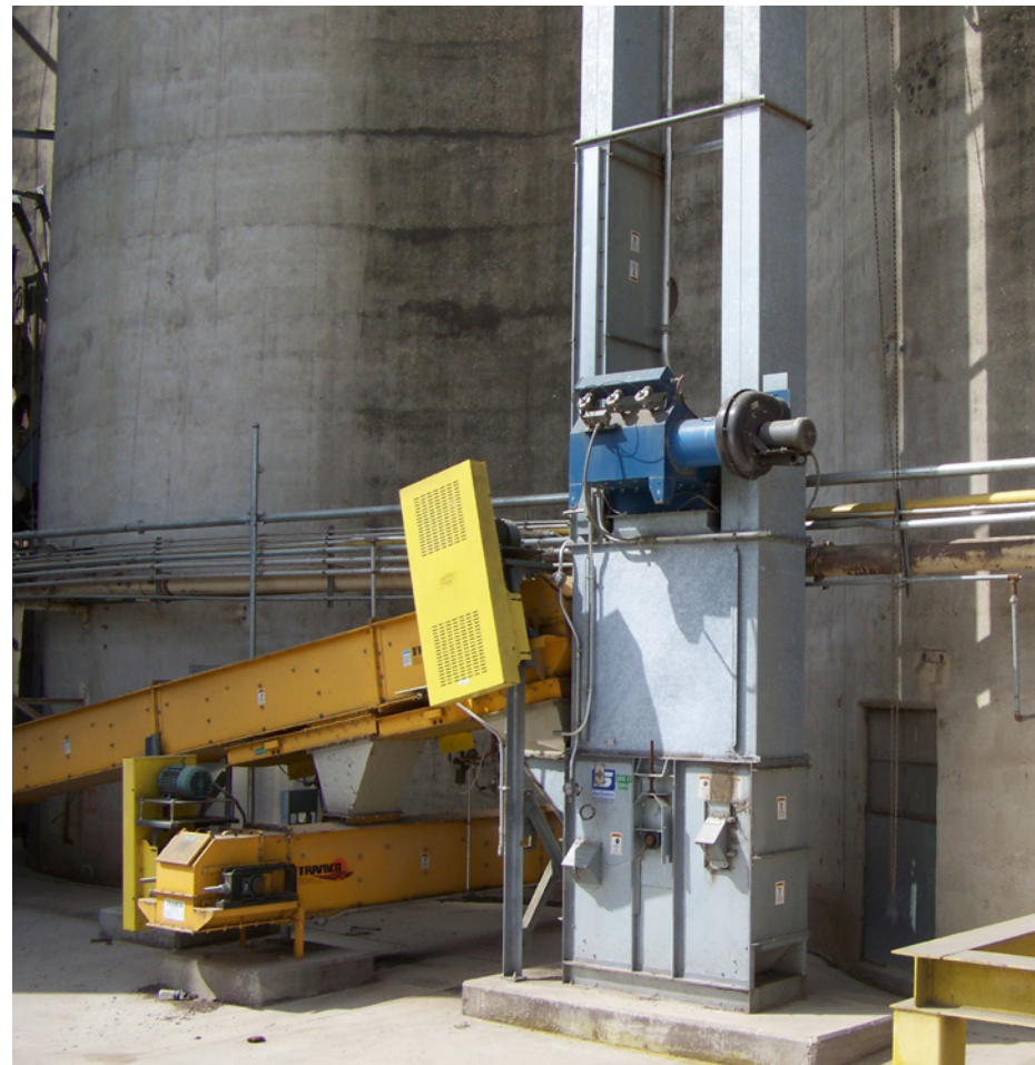
Figure 6. Point-of-Use Dust Control on Elevator Leg
