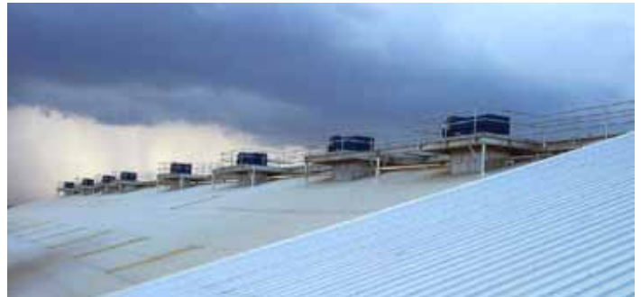
Donaldson Torit Dalamatric Insertables used as an integrated solution at Southern Cement.
