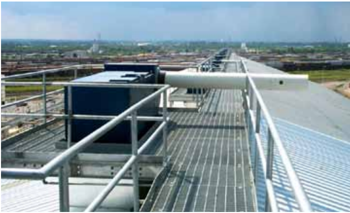
Donaldson Torit Dalamatric Insertable as integrated solution at Southern Cement.
