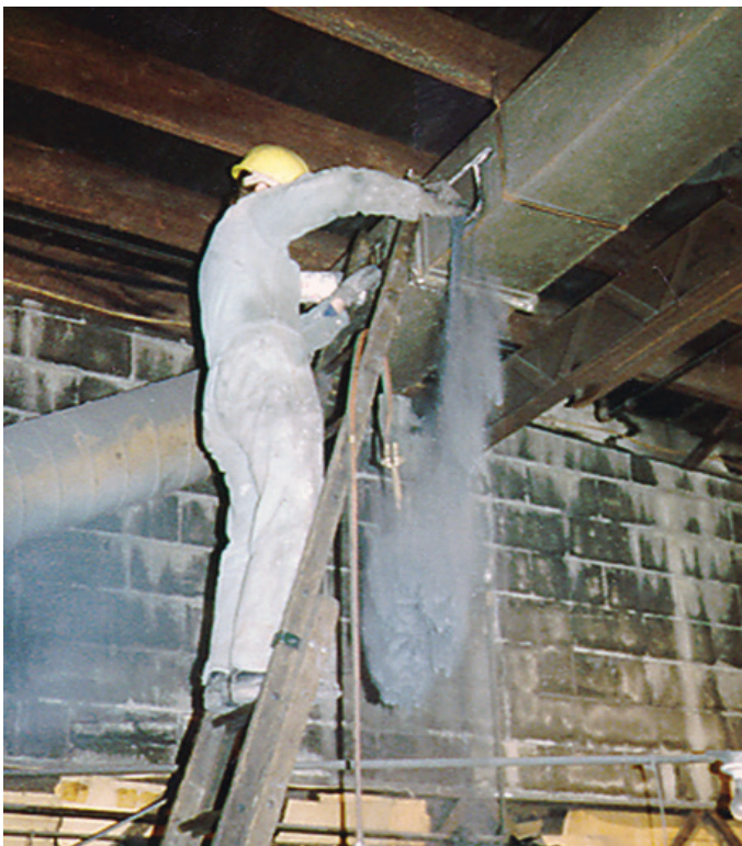
FIGURE 1 – To prevent the settling of dust within duct work, an appropriate conveying velocity is necessary.
